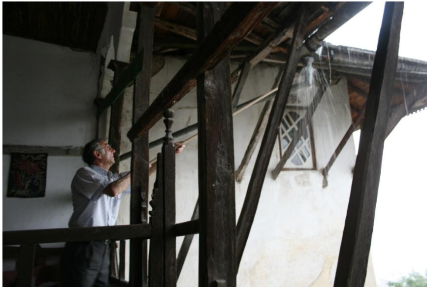
Figure 1: The owner of Skenduli House, turning aside the vertical pipe in order to avoid the water to go to the cistern. September, 2012
