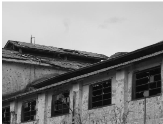
Figure 4 Electric central degradation.
