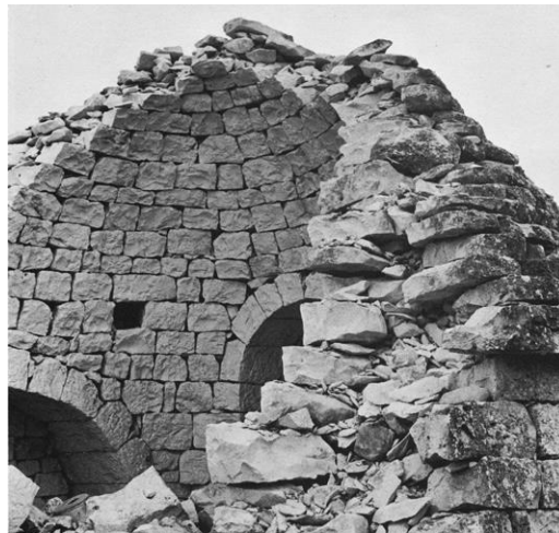
Fig. 3. Example of partial collapse of trullo vault [1]
