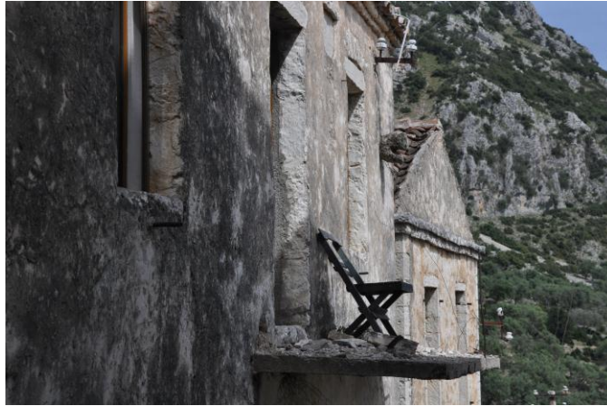
Figure 4. An abandoned house in Qeparo Village
