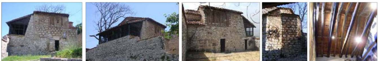
Fig. 19:View of present state of conservation of the church (elevations and structure of the roof)
