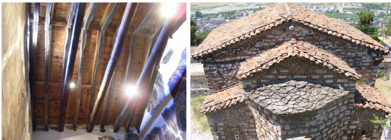
Fig. 7: View of the structure of the roof (left) and view of the roof (right)
