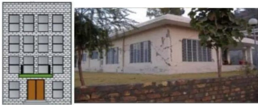
Figure 6. Immediate occupancy building performance level, moderate overall damage [3]
