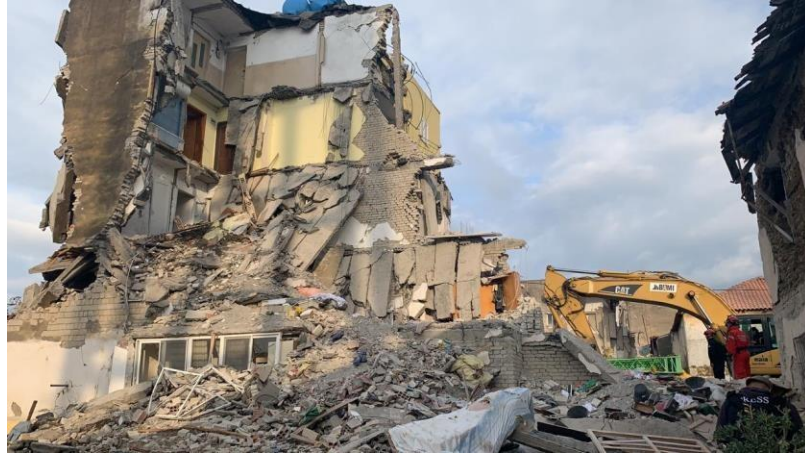
Figure 4. The structure collapsed in Thumanë [20]
