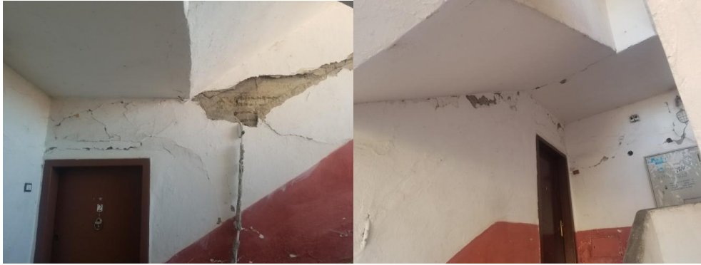
Figure 6. Presence of cracks in ramps
