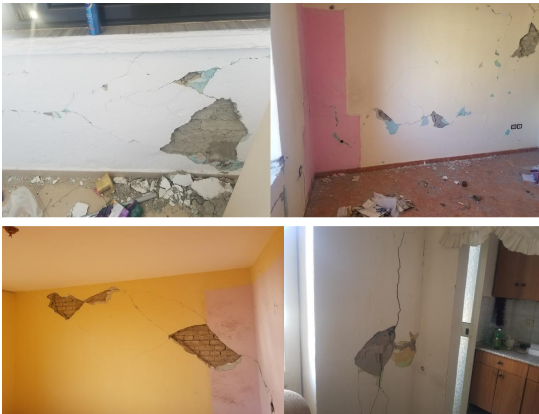
Figure 5. Cracks in the building with dimension more than 5 mm (1-4)
