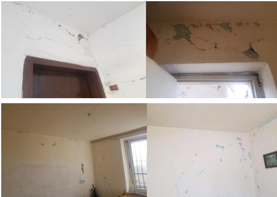
Figure 7. Cracks with dimension less < 5\text{ mm} near doors, windows
