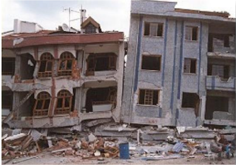
Figure 3 Buildings Pounding in 2009 New Zealand Earthquake (Khatami, Far, & Karimi, 2014)
