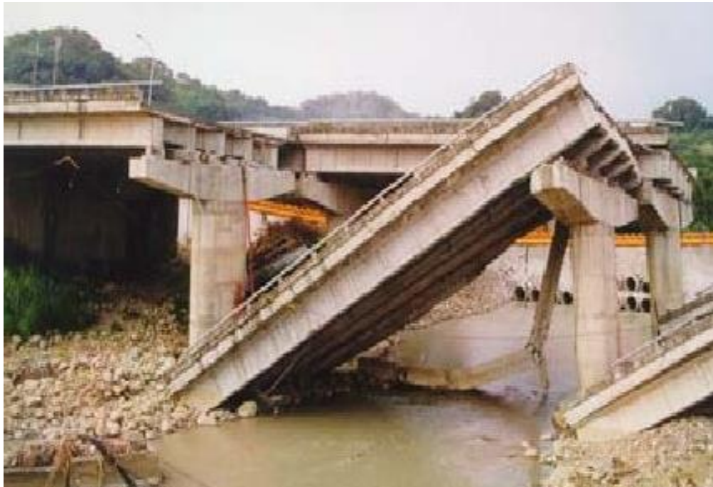
Figure 2 Bridge Pounding in 1999 Chi-Chi Earthquake (Sun, Li, Bi, Chow, Butterworth, & Hao, 2011)
