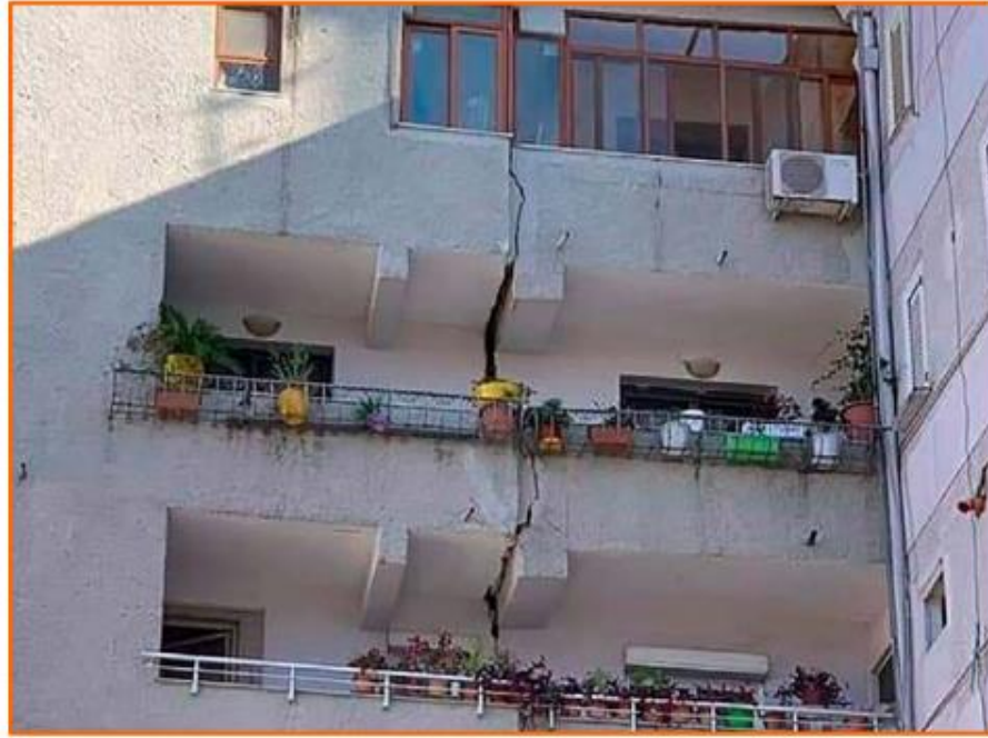
Figure 9 Pounding development in Tirana during Durres Earthquake of 2019 (Lekkas, Mavroulis, Filis, & Carydis, 2019)
