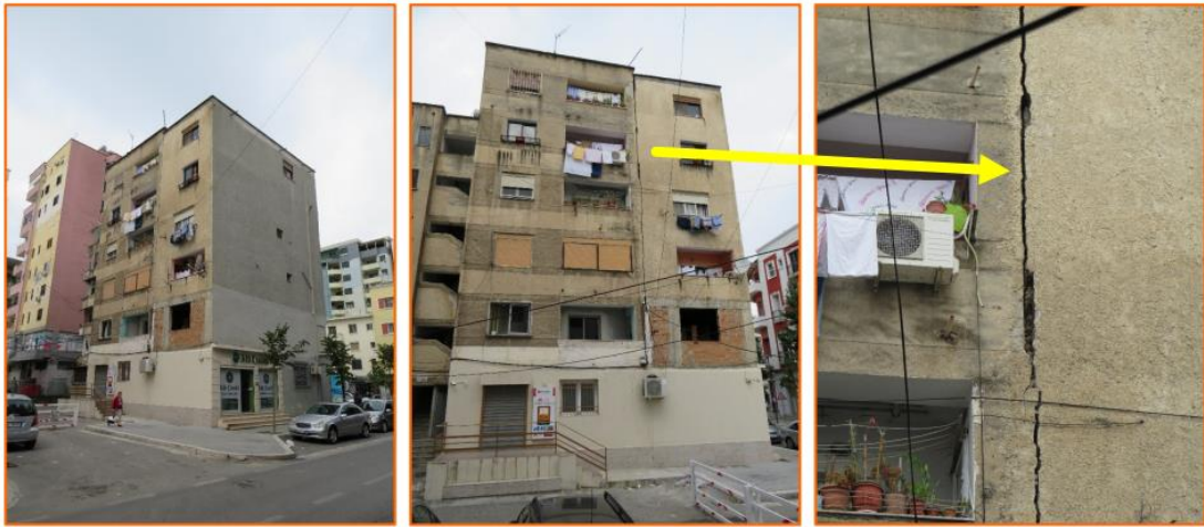
Figure 7 Pounding development due to the lowest mode of vibration in Durres Earthquake of 2019 (Lekkas, Mavroulis, Filis, & Carydis, 2019)
