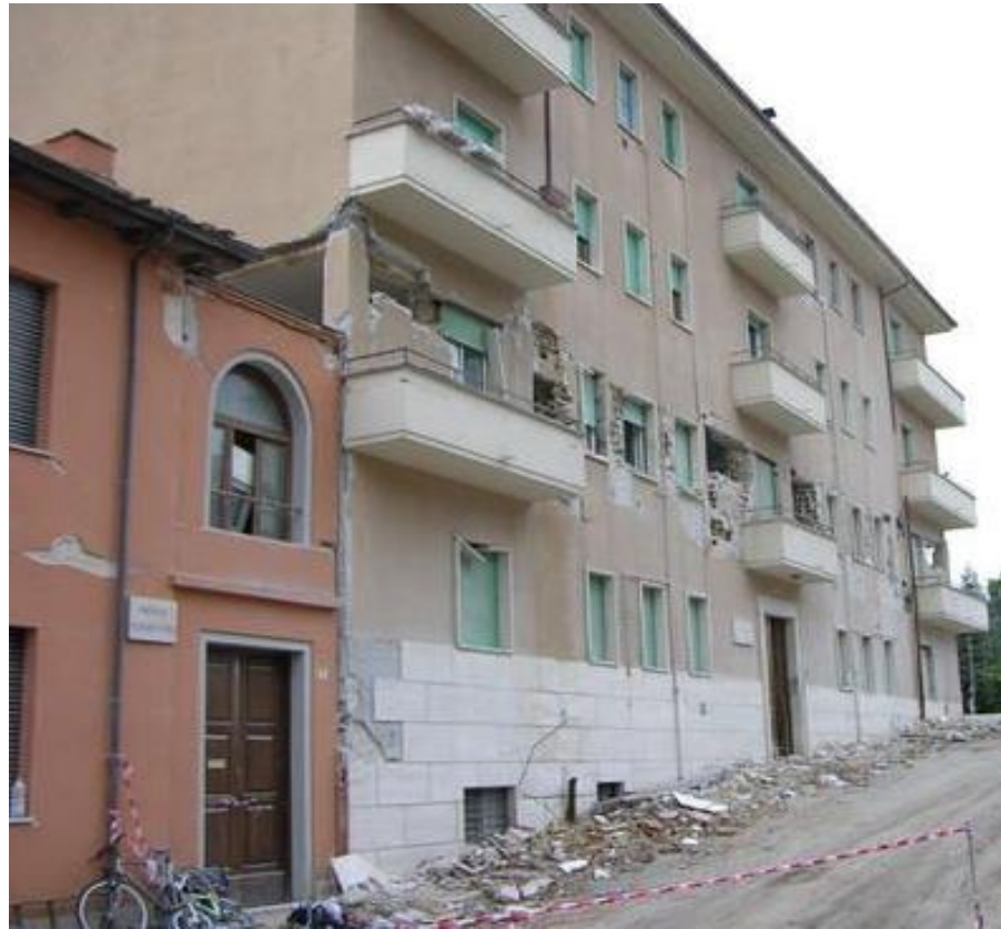
Figure 4 Buildings Pounding in 2009 L'Aquila Earthquake (Raheem, 2014)
