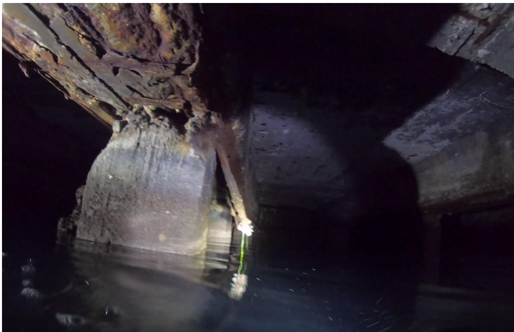
Figure 16 - Exposed heavily corroded reinforced bars at the apron's bottom and poor connection joint with the vertical pile - Quaywall 1.
