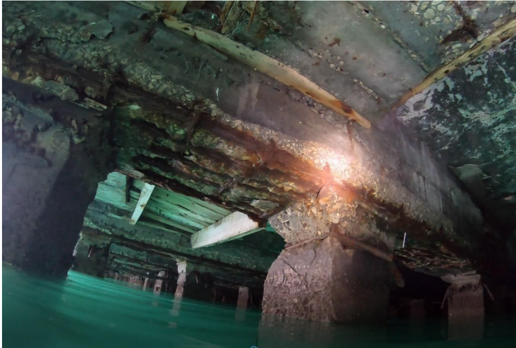
Figure 17 - Exposed heavily corroded reinforced bars at the apron's bottom - Quaywall 1.
