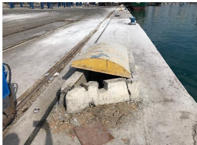
Figure 27 - Crane damaged power plug, on apron of quay 2
