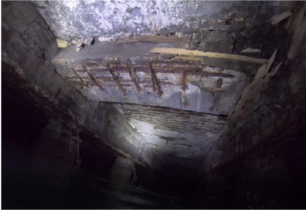
Figure 15 - Exposed heavily corroded reinforced bars at the apron's bottom of Quaywall 1.
