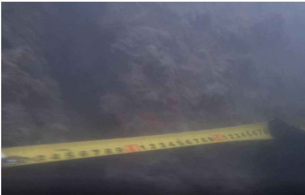
Figure 12 - Void between retaining piles of Quaywall 2
