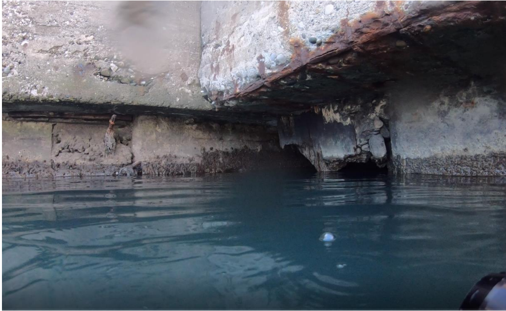
Figure 11 - Cavity at the joint between Quays 2 and 3. This damage may lead to filling material loss as mentioned before
