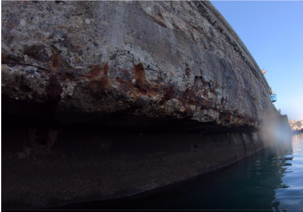
Figure 13 - Lightly damaged apron of Quaywall 2.
