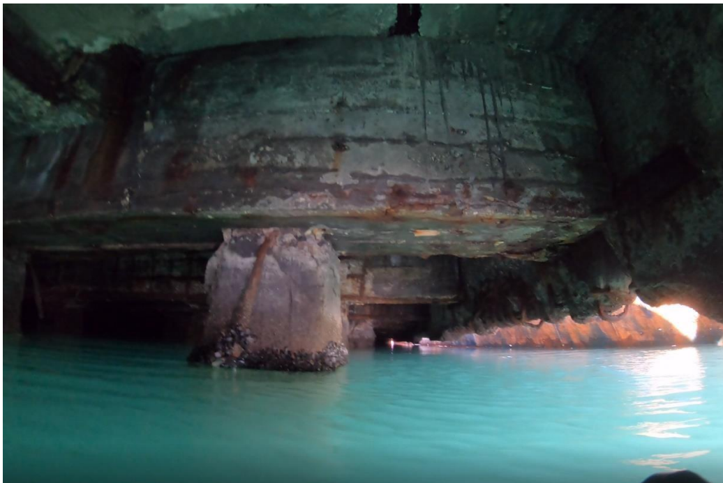
Figure 14 - Corrosion of RC structure
