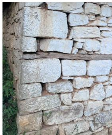
Figure 17. Wall system sketch and picture based on house found in Shëngjin village, owned by A.Myftari
