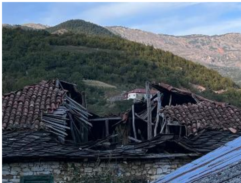
Figure 13. Demolished roof with exposed structure found in Shëngjin village, house owned by A.Myftari.
