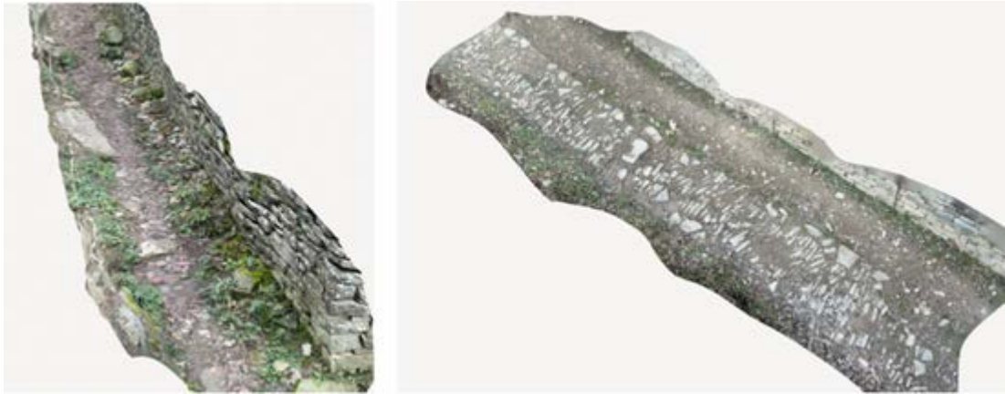
Figure 50. A 3D view of a section of road where the cobblestone pavement is severely damaged
