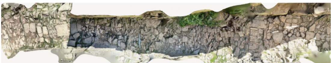
Figure 52. A 3D view of a section of road where the cobblestone pavement is in good state
