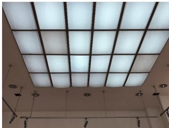
Figure 5. 12/b The state of the ceiling now.
