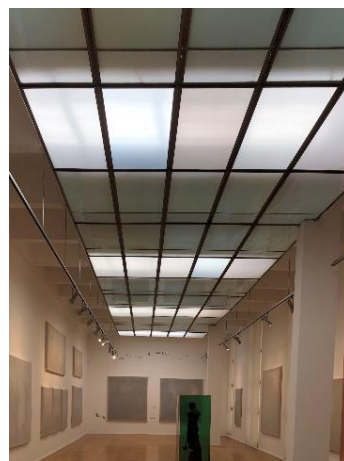
Figure 5. 13/b The state of the ceiling now.
