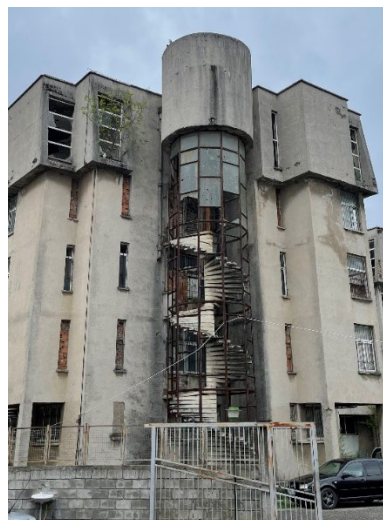
Figure 22. Picture of the former psychiatric building, which was rapidly depreciating due to lack of maintenance.
