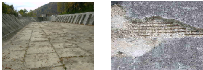
Fig.2. The view of the accumulations basin and degradation of concrete in concrete campades
