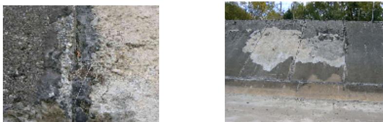
Fig.2. The joint connection between the floor and wall; joint between the concrete campades
