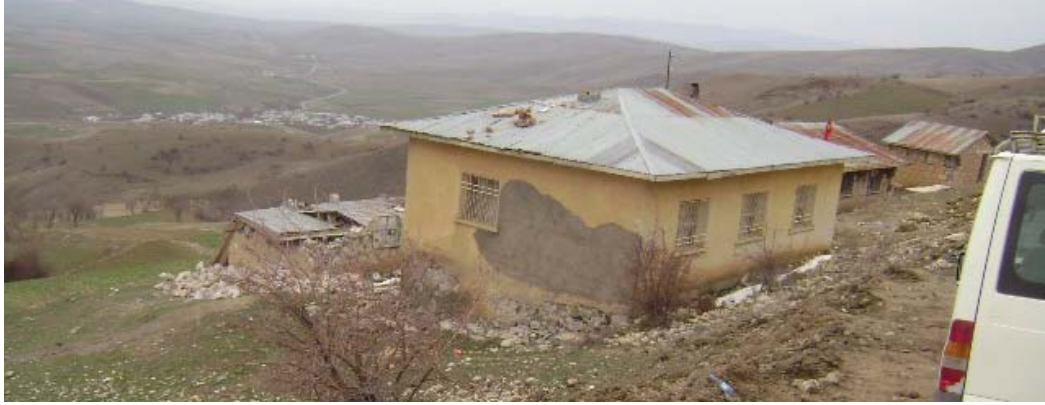
Figure 10 Many of the damaged buildings were located on the hills with a high slope
