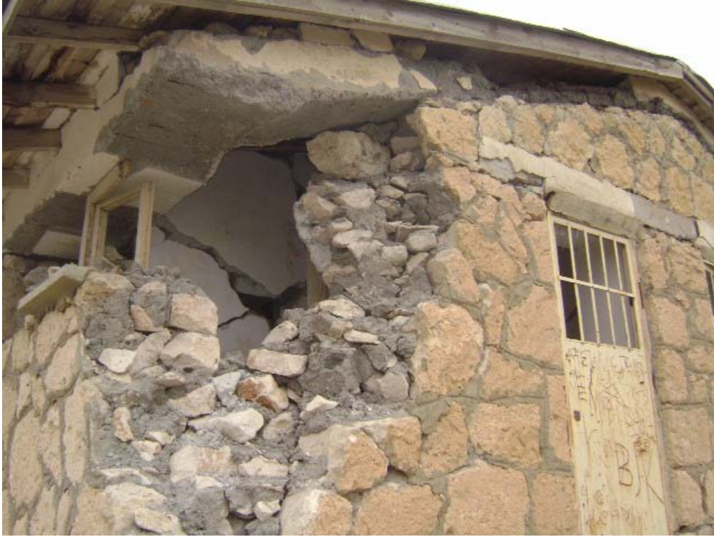
Figure 4 Rubble stone and shaped soft stone blocks used as the wall materials
