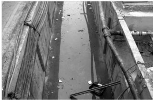
Figure 8: An infrastructure tunnel with destroyed top-cover and filled with water (Canto-Perello and Curiel-Esparza, 2006)
