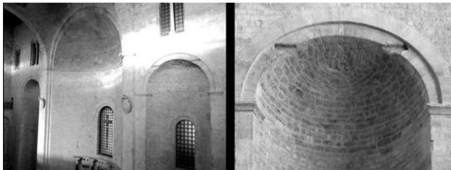
Figure 1: Apsidal vaults in Basilica of St. Nicholas in Bari. The case of study is on the right
